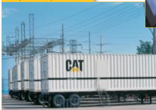
Multiple Backup Gensets
